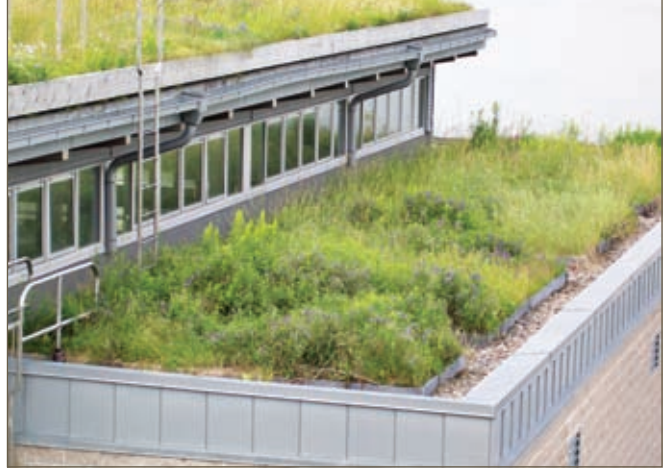
Pictured above, the extensive green roof at the Bedford Oceanography Institute in Dartmouth, N.S., was installed in 2002. The assembly consists of a wide variety of grasses.
